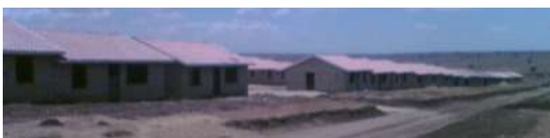
A new town under construction in Kajiado district central Kenya constructed almost entirely with Parry technology. This project like many others around the world has depended on Parry innovation and knowledge.
