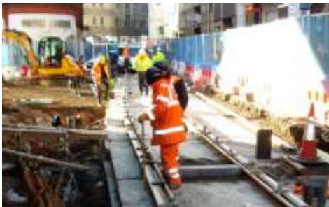
Work on extension of the electrified Midland Metro system has caused serious disruption to Birmingham city centre for over a year
